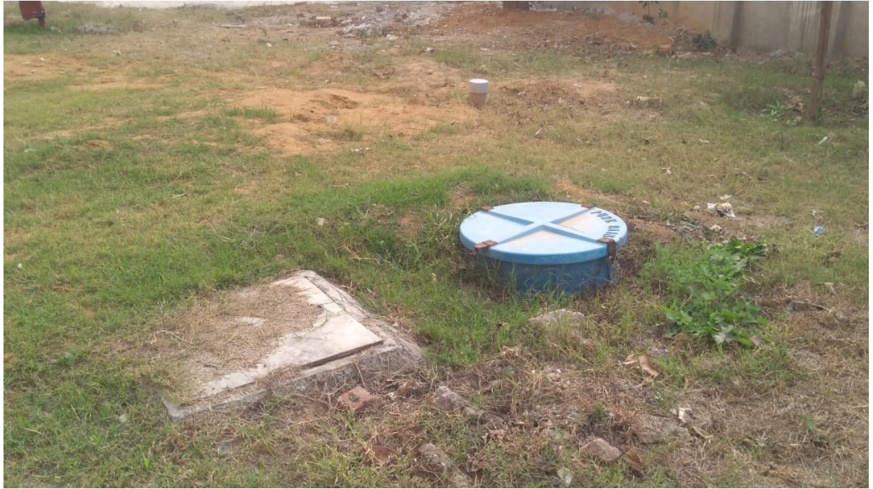
D Block (Paramedical Block) back side Rainwater harvesting pit
