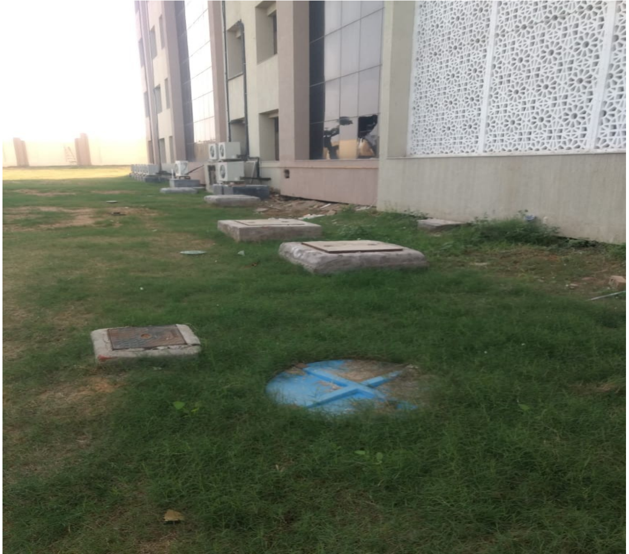
A Block back side Rainwater harvesting Pit
